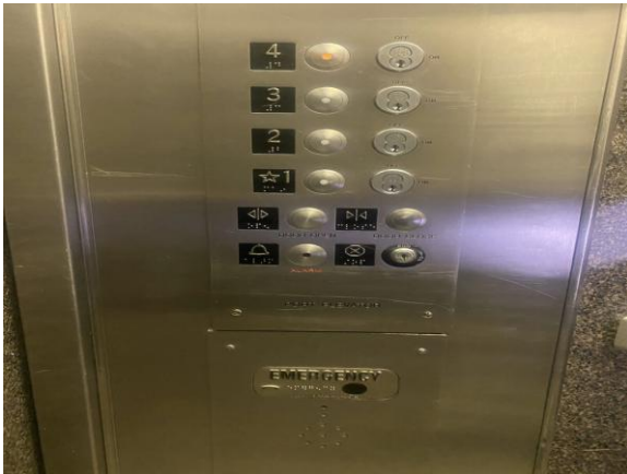
0013-000001a 1/30/2025 Elevator panel Elevator
