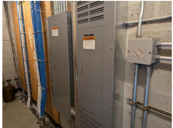
0013-000020e 1/30/2025 Electrical distribution panel PP3 Room 418
