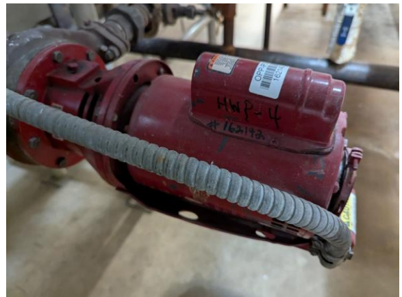
0013-000042e 1/30/2025 Domestic hot water pump HWP-4 Room M001
