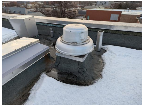
0013-000001e 1/30/2025 Centrifugal curb-mounted exhauster EFN-007 Roof
