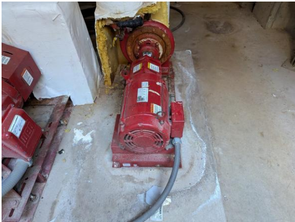
0013-000051e 1/30/2025 Chilled water pump CHWP-3 Room M002
