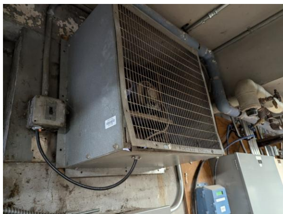
0013-000046e 1/30/2025 Louvered propeller style exhaust fan EF-1 Room M001
