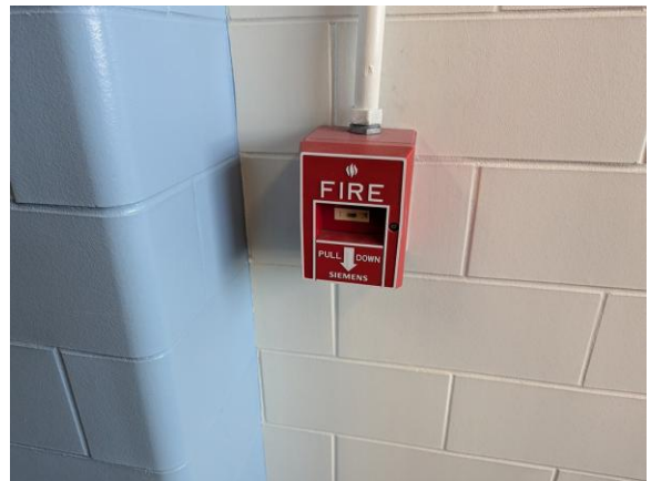
0013-000014e 1/30/2025 Fire alarm manual pull station Corridor Q401
