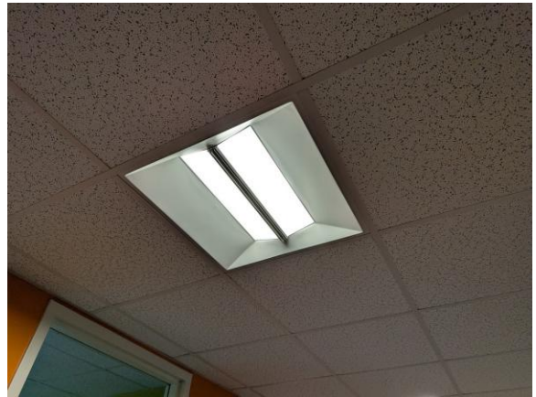
0013-000019e 1/30/2025 Lay-in LED fixture Room 422
