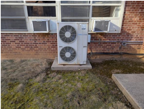
0013-000049e 1/30/2025 Air-cooled condenser for ductless split system CU-3 Courtyard
