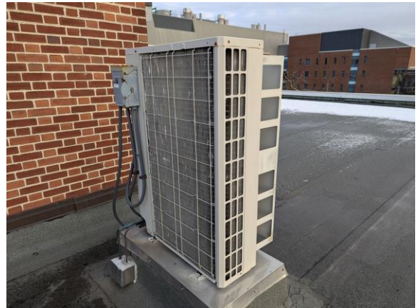
0013-000005e 1/30/2025 Air-cooled condenser for ductless split system CU-1 Roof
