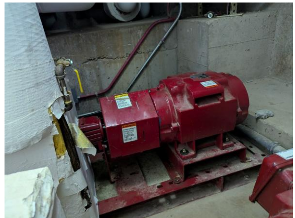
0013-000054e 1/30/2025 Heating water pump HWP-4 Room M002
