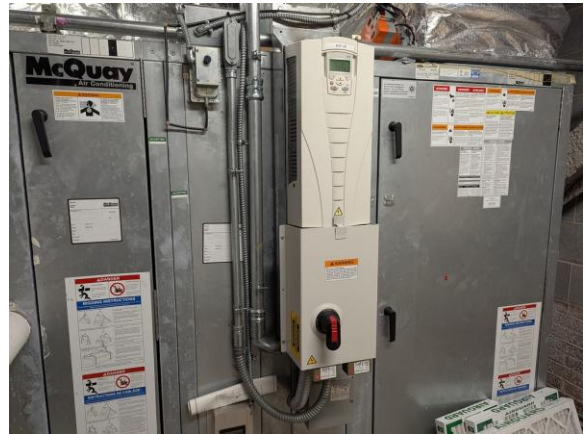
0013-000022e 1/30/2025 Variable frequency drive VFD AHU-3 Room M325
