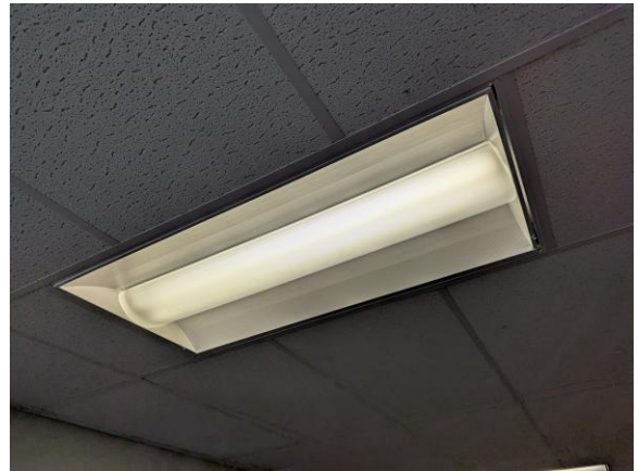
0013-000013e 1/30/2025 Lay-in fixture with T8 fluorescent lamps and acrylic prismatic lens Corridor Q401
