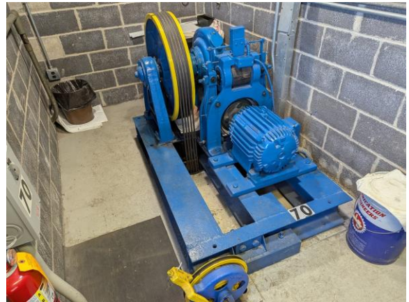
0013-000010e 1/30/2025 Traction mechanism for passenger elevator 070 Room M501
