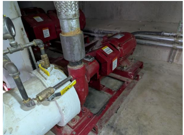
0013-000052e 1/30/2025 Heating water pump HWP-6 Room M002
