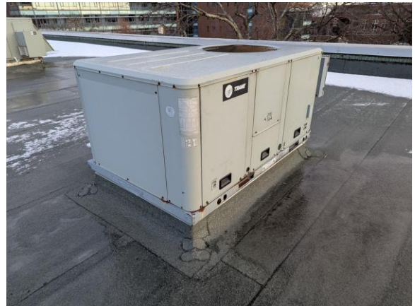
0013-000002e 1/30/2025 Package air conditioning unit RTU-5 Roof
