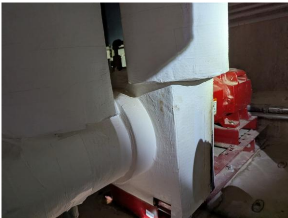
0013-000053e 1/30/2025 Heating water pump HWP-5 Room M002
