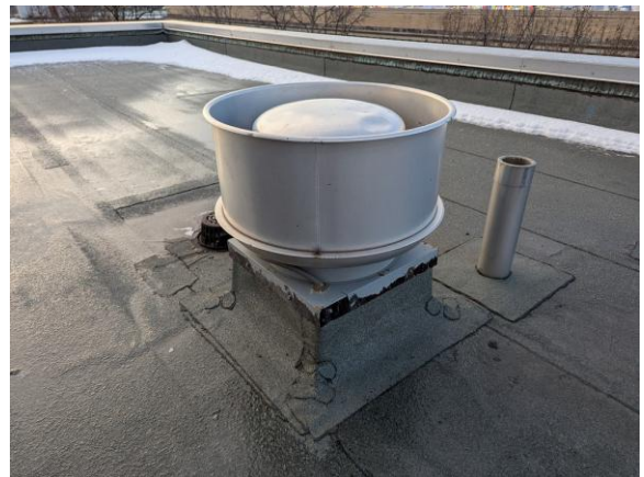
0013-000009e 1/30/2025 Centrifugal curb-mounted exhauster EFN-005 Roof
