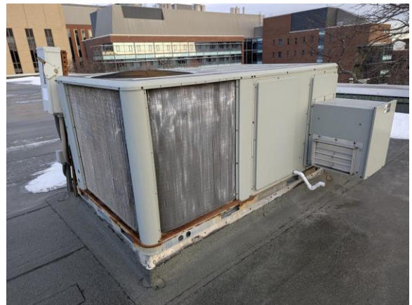
0013-000003e 1/30/2025 Package air conditioning unit RTU-1 Roof
