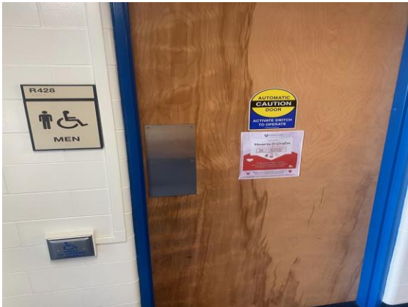
0013-000011a 1/30/2025 Power-assisted door operator Restroom
