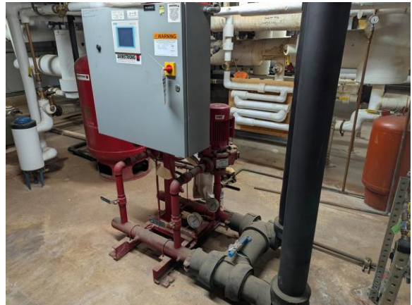
0013-000038e 1/30/2025 Duplex domestic water booster pump skid BP-1 Room M001
