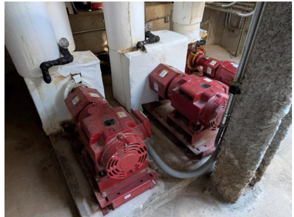
0013-000050e 1/30/2025 Chilled water pumps CHWP-1 and CHWP-2 Room M002
