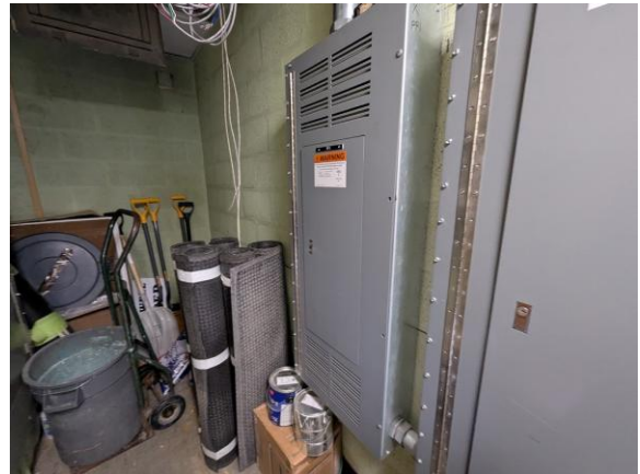
0013-000029e 1/30/2025 Electrical distribution panel PP1 Room P115
