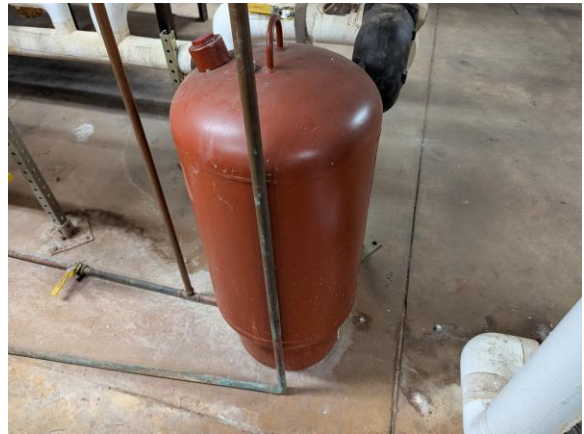
0013-000037e 1/30/2025 Heating water expansion tank ET-HHW-1 Room M001
