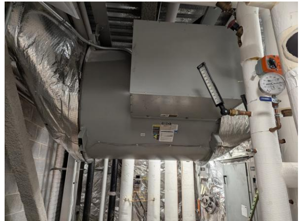
0013-000023e 1/30/2025 Axial flow return air fan RF-3 Room M325
