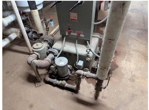
0013-000041e 1/30/2025 Duplex condensate receiver CP-1 Room M001
