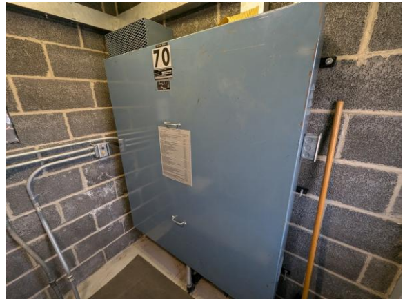
0013-000011e 1/30/2025 Solid state control panel for passenger elevator 070 Room M501
