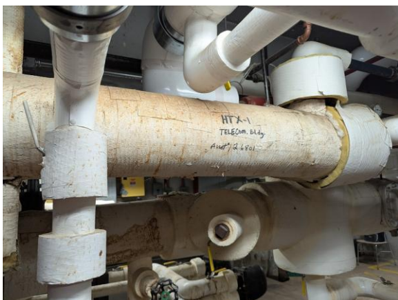
0013-000043e 1/30/2025 Shell-and-tube heat exchanger serving Telecom Building (HTX-1) Room M001
