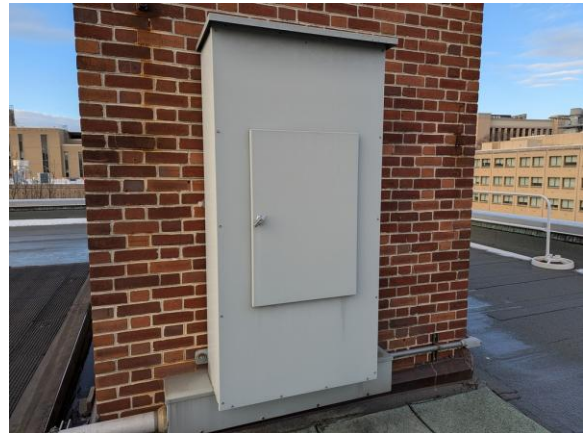
0013-000008e 1/30/2025 Electrical distribution panel Roof
