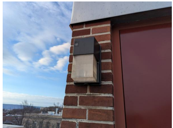
0013-000012e 1/30/2025 LED wall pack Roof
