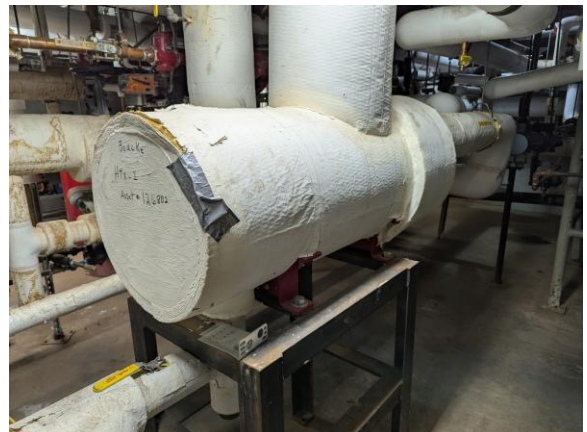
0013-000036e 1/30/2025 Shell-and-tube heat exchanger HTX-2 Room M001
