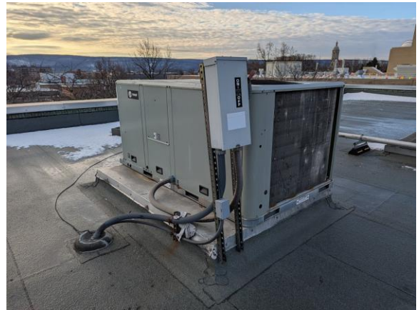
0013-000007e 1/30/2025 Package air conditioning unit RTU-2 Roof
