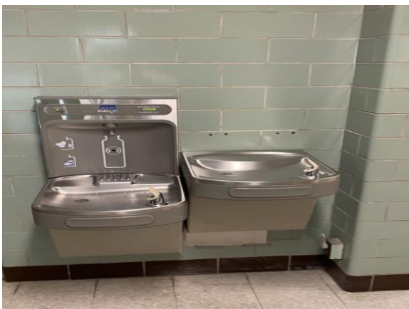
0013-000030a 1/30/2025 Dual-level drinking fountain Corridor
