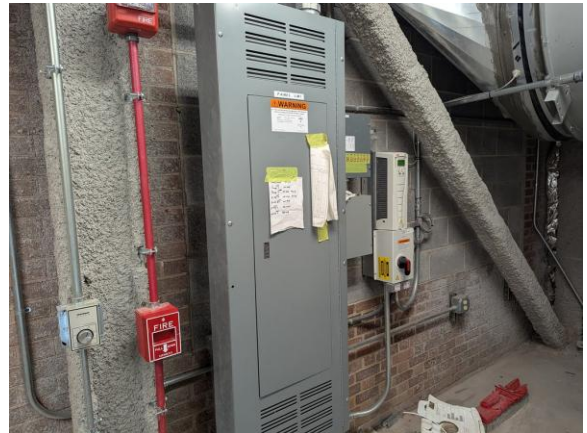
0013-000035e 1/30/2025 Electrical distribution panel LM1 Room M140
