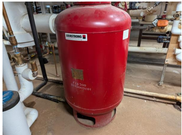
0013-000039e 1/30/2025 Domestic water expansion tank ET-1, DCW Room M001
