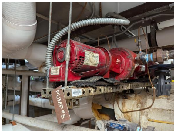
0013-000044e 1/30/2025 Heating water pump serving Telecom Building (HWP-006) Room M001
