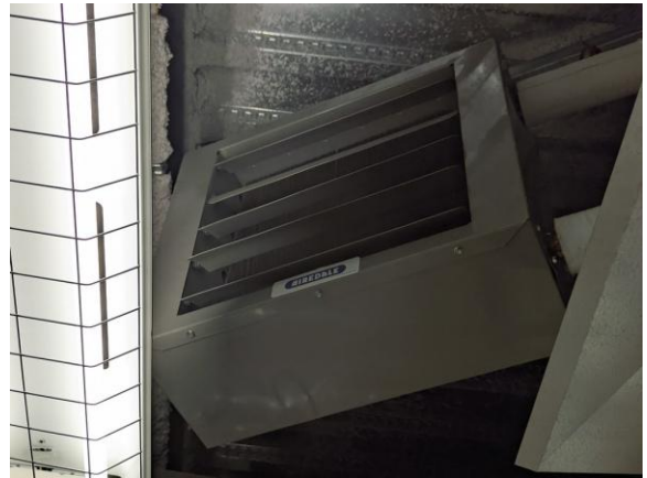
0013-000034e 1/30/2025 Hydronic unit heater UH-2 Room M140
