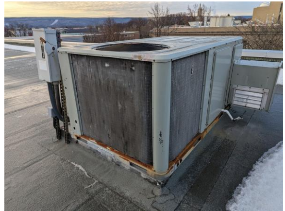
0013-000004e 1/30/2025 Package air conditioning unit RTU-4 Roof
