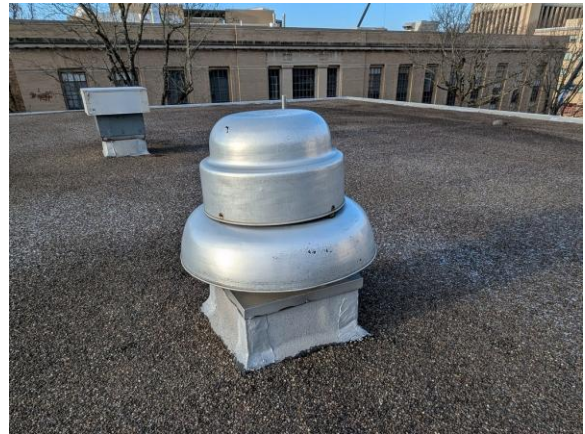
0013-000016e 1/30/2025 Centrifugal curb-mounted exhauster EFN-002 Lower roof
