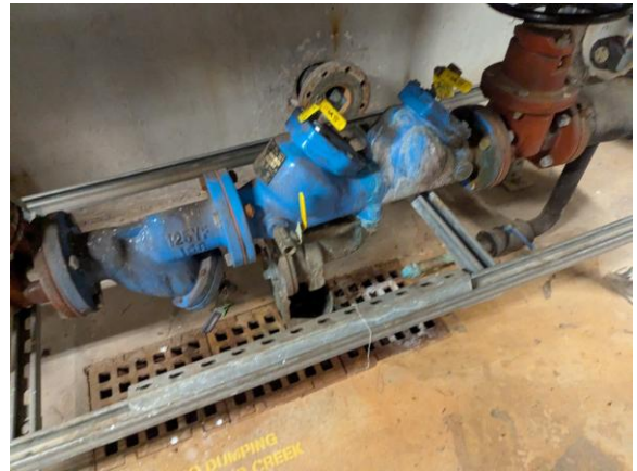
0013-000040e 1/30/2025 Backflow preventer Room M001
