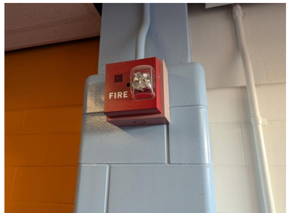
0013-000015e 1/30/2025 Fire alarm horn and strobe signaler Corridor Q401
