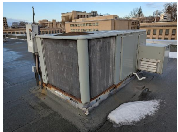
0013-000006e 1/30/2025 Package air conditioning unit RTU-3 Roof
