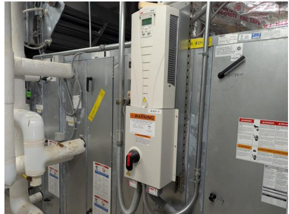
0013-000031e 1/30/2025 Variable frequency drive VFD AHU-1 Room M140
