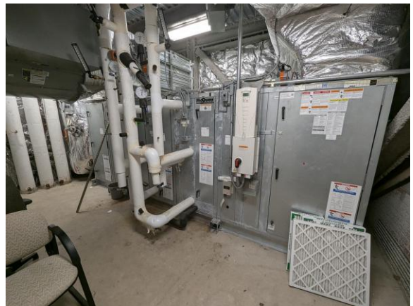
0013-000021e 1/30/2025 Indoor air handler AHU-3 Room M325
