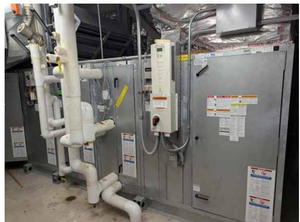
0013-000030e 1/30/2025 Indoor air handler AHU-1 Room M140
