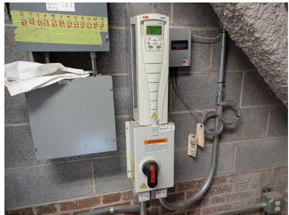
0013-000033e 1/30/2025 Variable frequency drive VFD RF-1 Room M140
