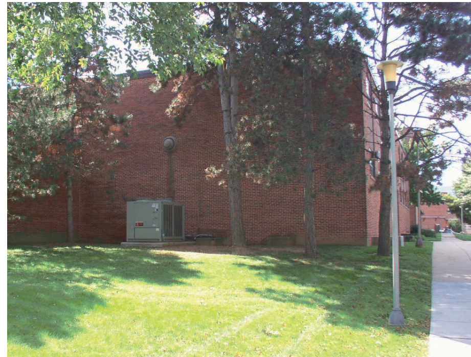
2 -Screen mechanical equipment
