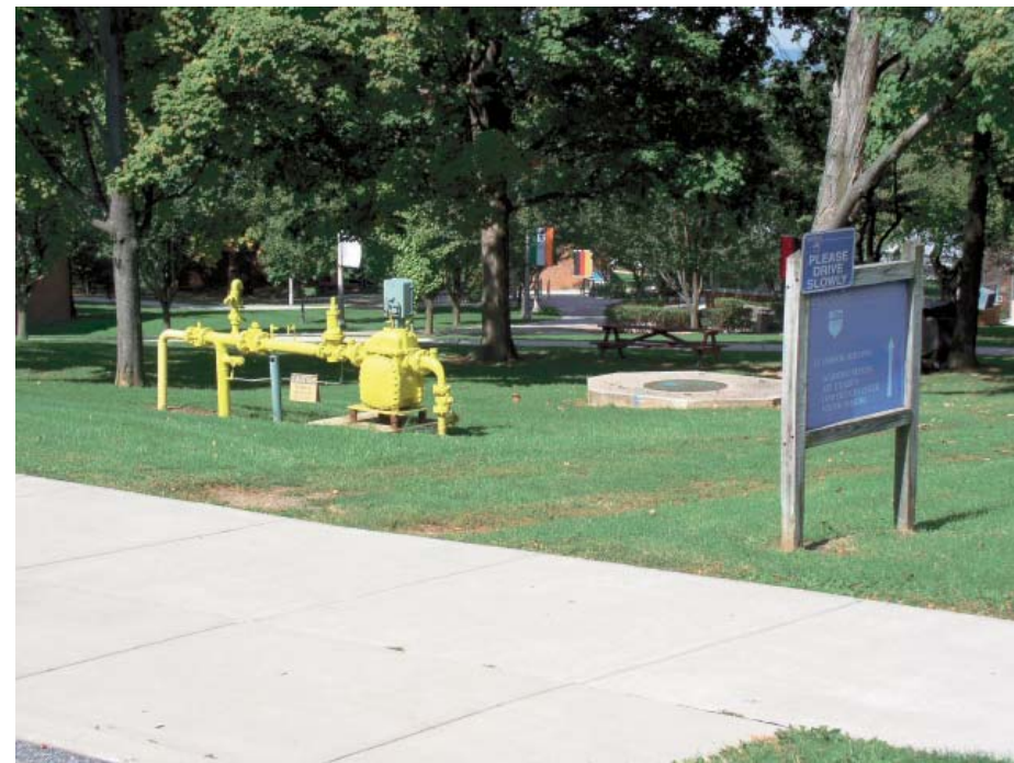
3 -Screen utility meters
