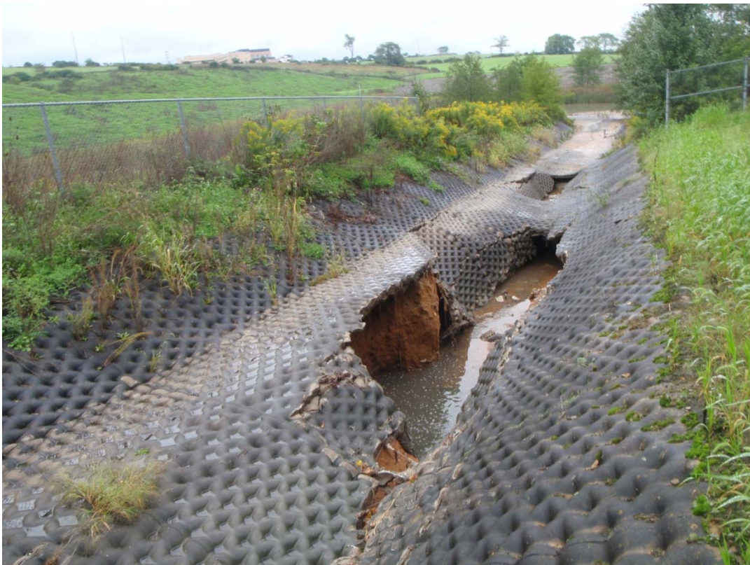
Figure 8.d Sinkhole under the Inflow Fabri-Form Concrete Channel
