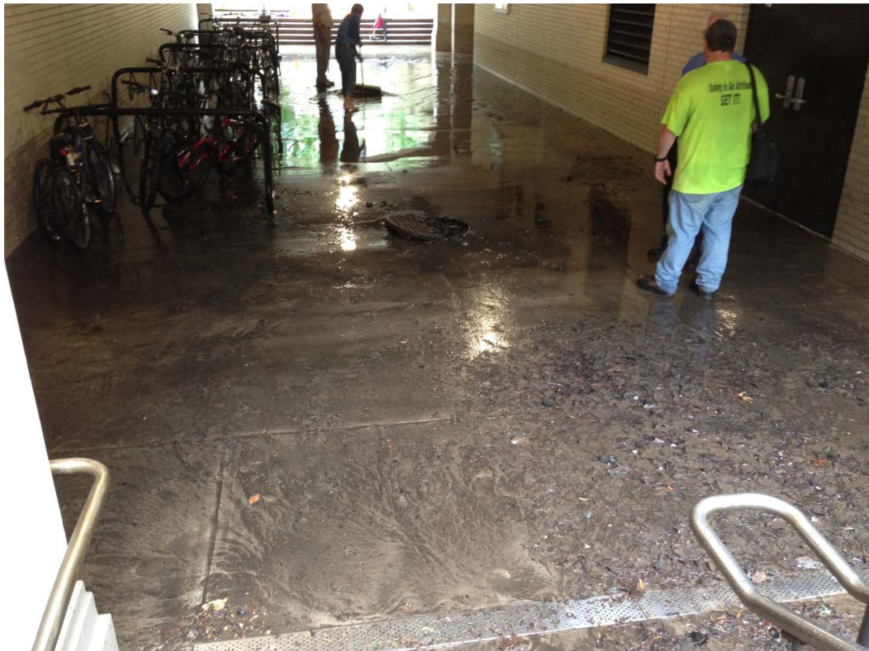
Figure 6.q. The Pattee Tunnel after Flooding 2 feet Deep on 6/25/2014
