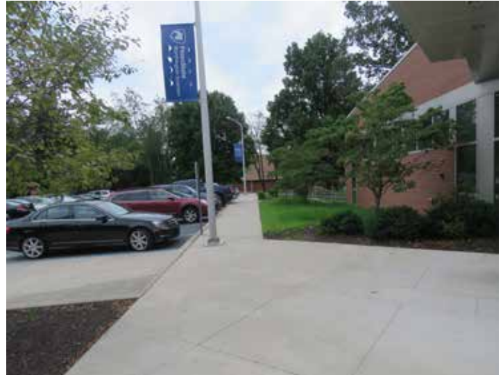
Non-standard parking lot light fixtures at Business parking lot
