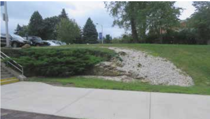
Dry-laid stone out of character and deteriorating
