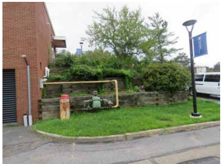
Utility pipes and meters are unsightly
