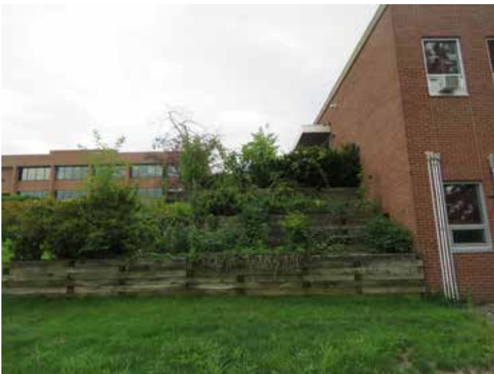
Timber walls are unattractive and not long-term solution
