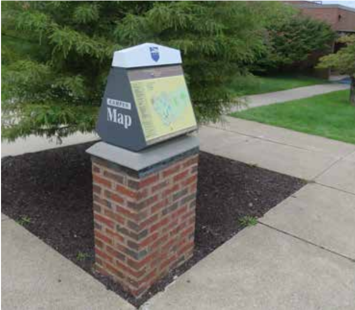
Replace way-finding sign panels because of deterioration
