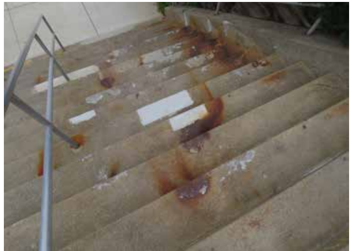
Close up view of patchwork repairs and ongoing decay
