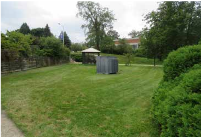
Exposed transformers are unattractive and distracting
