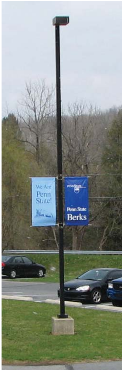
Parking Lot/Roadway Light
