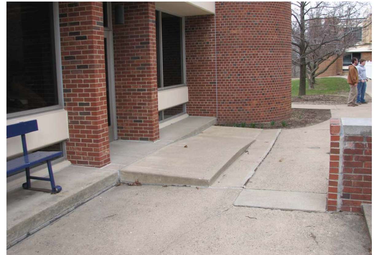
Hazardous tripping conditions should be eliminated
