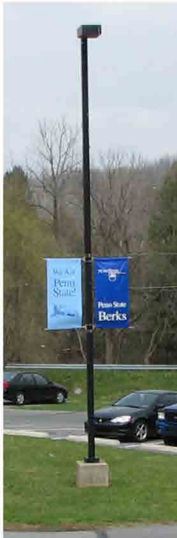
Parking Lot/Roadway Light
